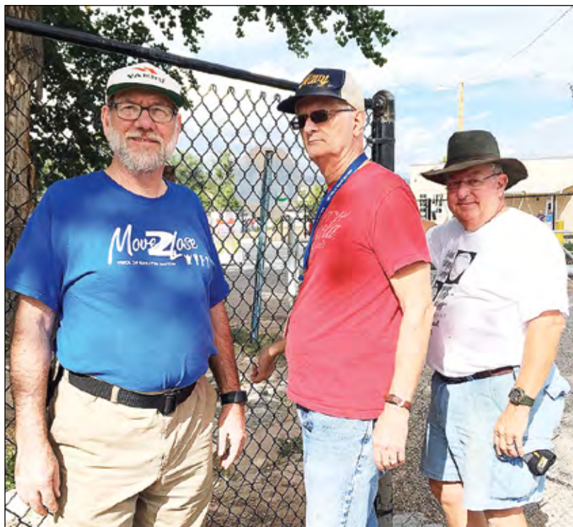
Above: Ohio volunteers from Sulphur Grove UMC are installing a fence. Below: Screen shot of the February 2019 McCurdy Volunteer News which is emailed on a monthly basis.
