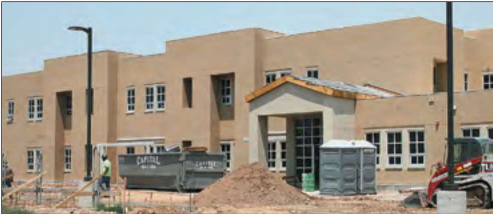
The outside of the charter school building is complete, outside lighting has been installed and the parking lot is being worked on.
