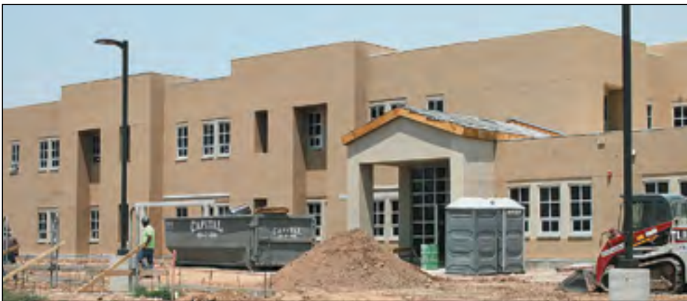
The outside of the charter school building is complete, outside lighting has been installed and the parking lot is being worked on.
